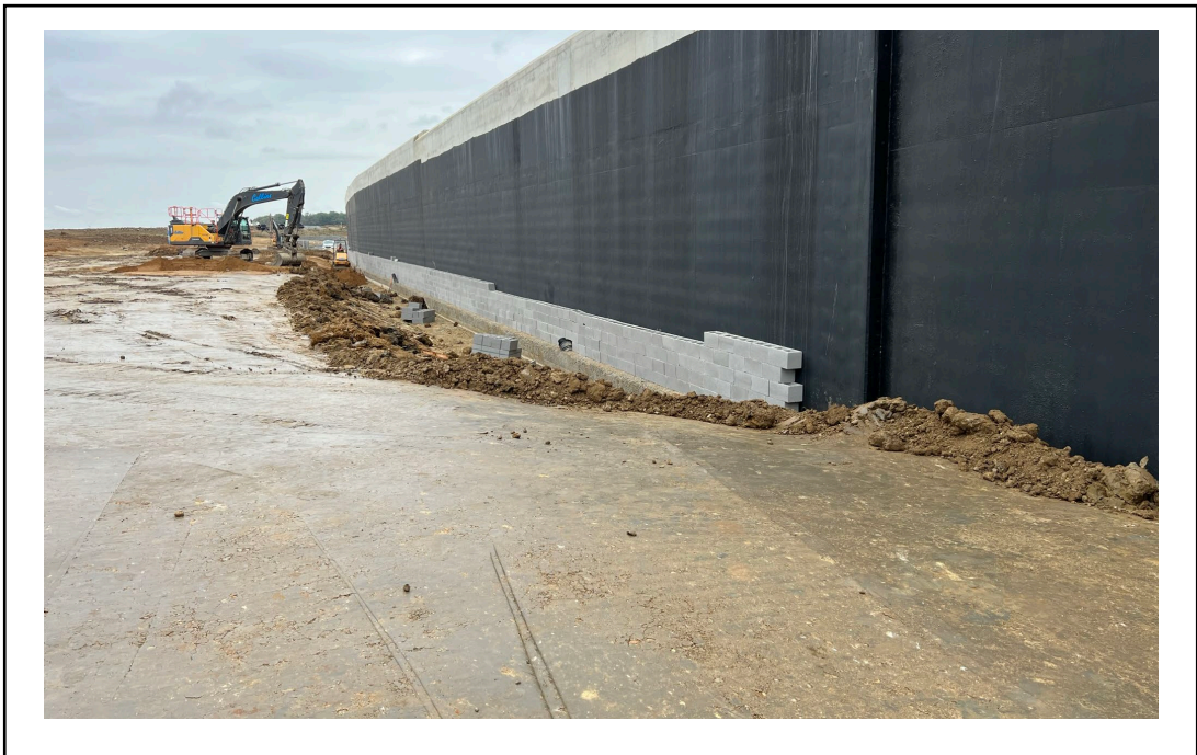
Photo 4 – Eastern side to Tunnel – earthworks and back of the wall drainage blocks installation
