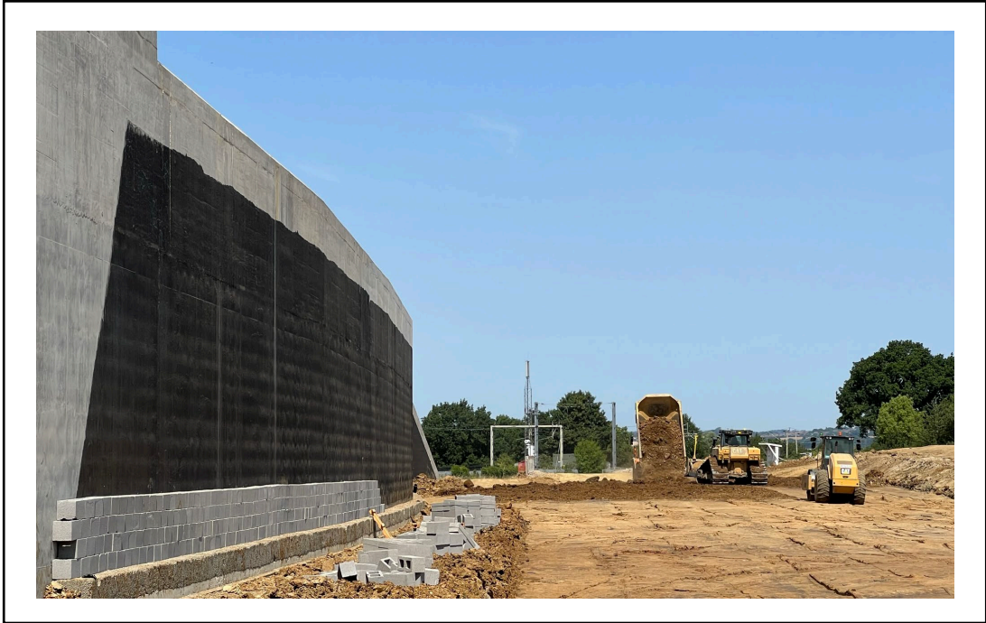
Photo 3 – Eastern side to Tunnel – earthworks and back of the wall drainage blocks installation
